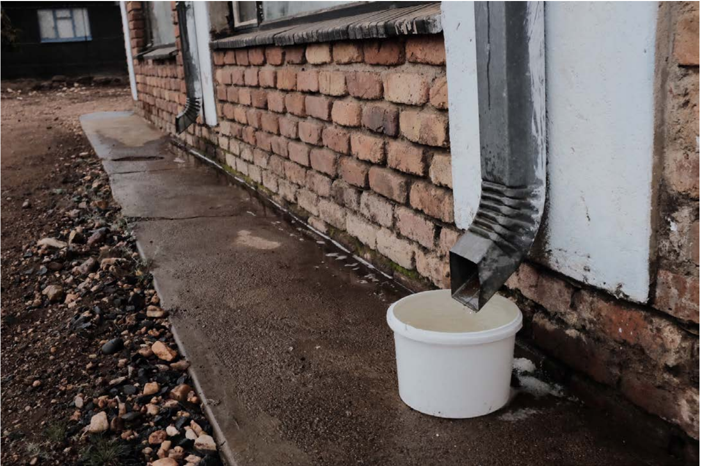
Homeowners in Siyandhani Village use downpipes on the side of the house to collect rain water, Siyandhani Village is close to the the town of Giyani in Limpopo Province. The province was declared a disaster area in 2015 due to ongoing droughts. Photo: Tim Moolman, Tim Moolman photography
